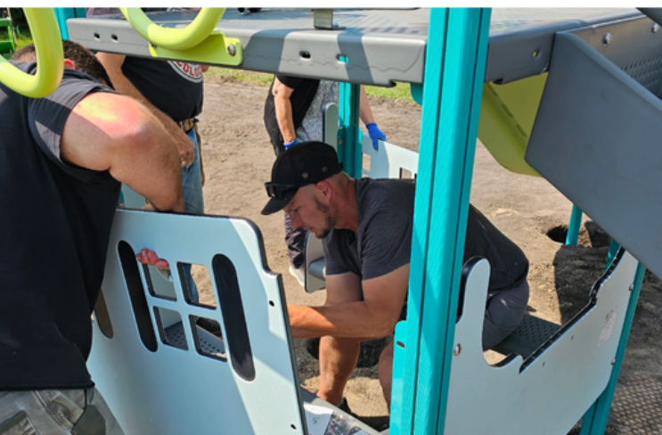
Volunteers installing new playground structures at Peony Farm Community Club, Portage la Prairie, MB
